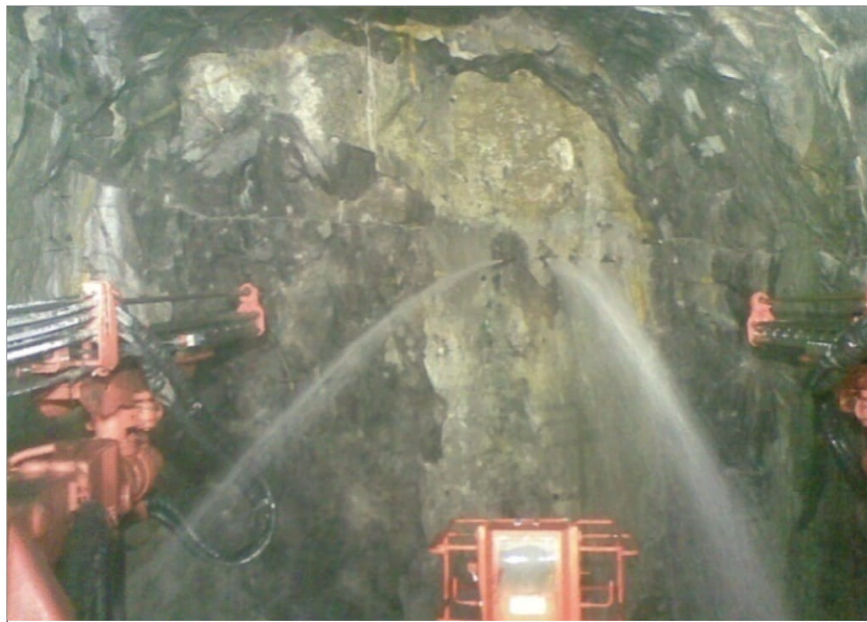
Figure 1: Water ingress during excavation
