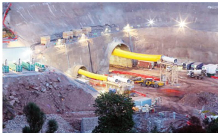
Fig. 1 - A view of Chenani-Nashri main tunnel and adjoining escape tunnel (photo: dailyexcelsior.com)
