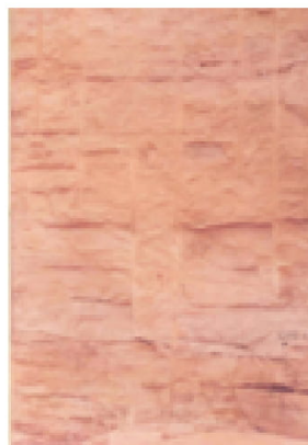
Fig. 23: Horizontal joints at RAPP units 3 and 4
