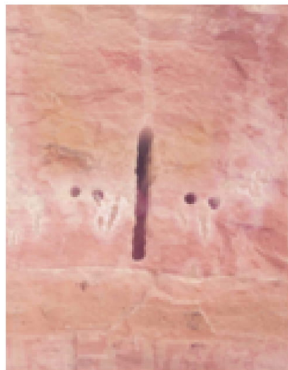
Fig.25: View of slot cut in the vertical direction at RAPP units 3 and 4
