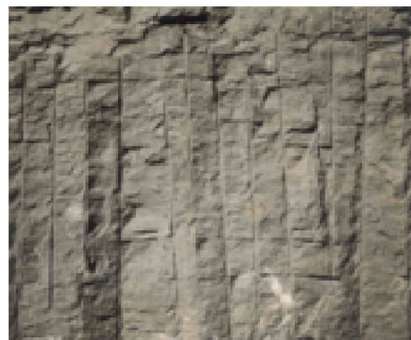
Fig. 24: Vertical joints at RAPP units 3 and 4
