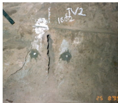
Fig. 4 - Slot cut in vertical direction to measure induced stress along the tunnel axis
