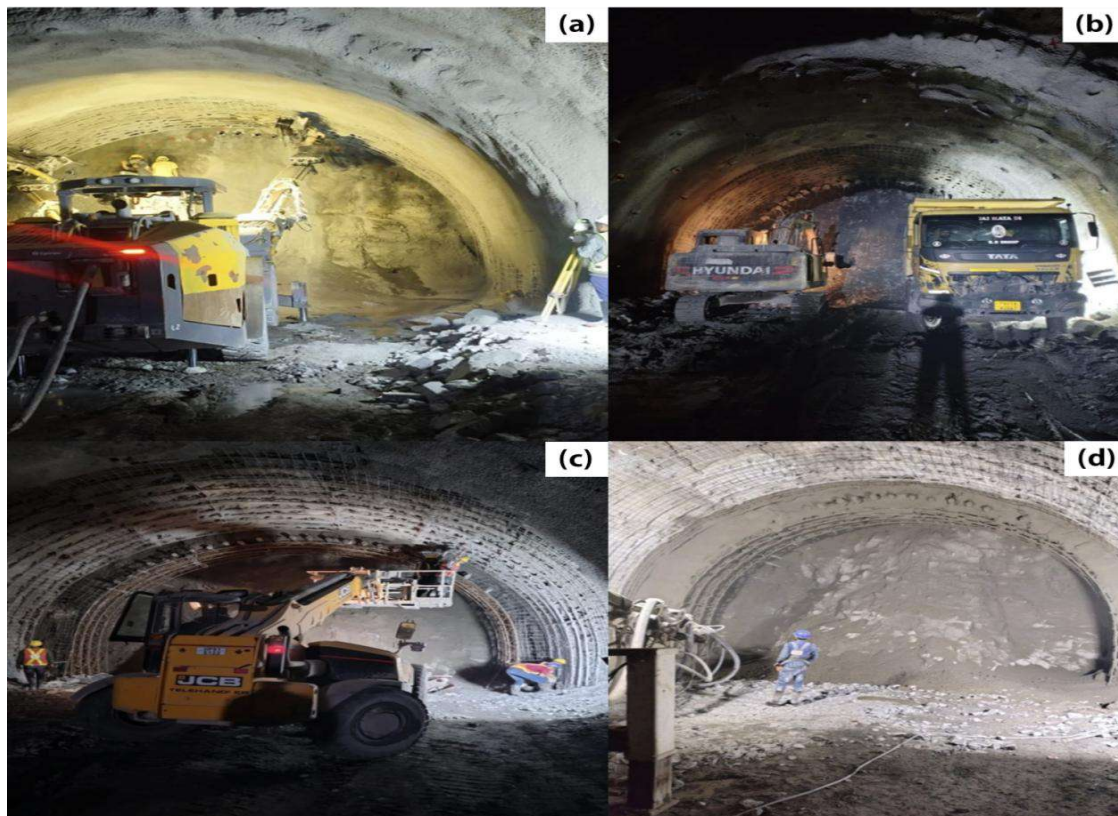
Figure 6- Construction process & support system (a) Piperoof Installation (b) Face Excavation & Mucking (c) Lattice Girder Erection (d) Shotcrete Application
