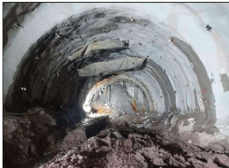
Figure 11- Face water seepage diverted in the already identified water seepage zone
