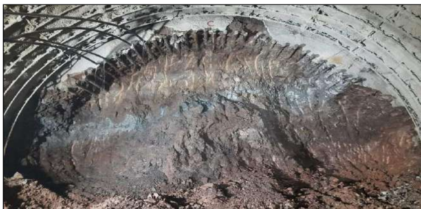
Figure 9- Water seepage during pipe roofing at Chainage 24+394.315m and diverted
