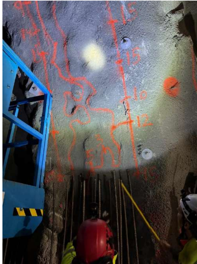
Figure 8 - Photo of a part of the temporary RRS2 that needed to be scaled down to fit the permanent support
