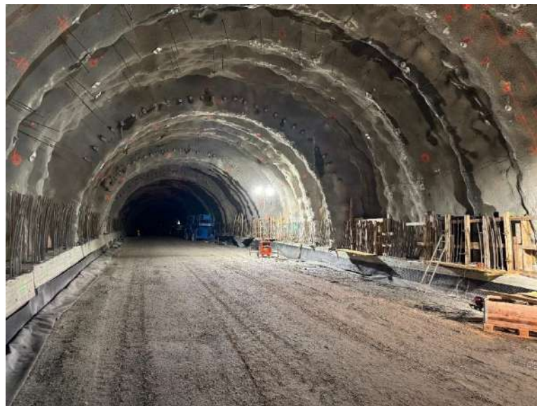
Figure 7 - Photo of the temporary support of Bergåsen tunnel, before the permanent RRS support
